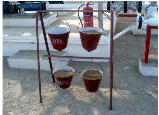
Sand buckets placed at various locations in the facility.
