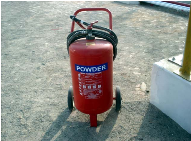
Trolley mounted fire extinguishers at various locations in the facility
